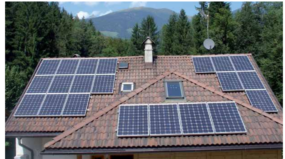
Elpo | Ehrenburg - Germany System: 5,04 kW | Roof fastener system
